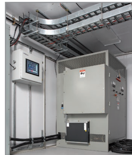
Hydrogen Generator Power Supply
